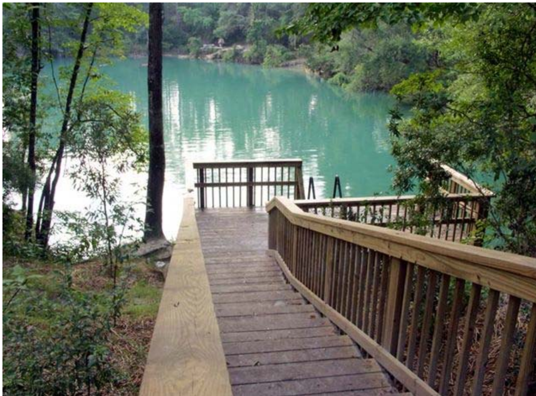
These steps were built over the eroded bank to prevent further erosion of soil into Cherokee Sink in Wakulla Springs State Park. Photo from Florida Park Service
